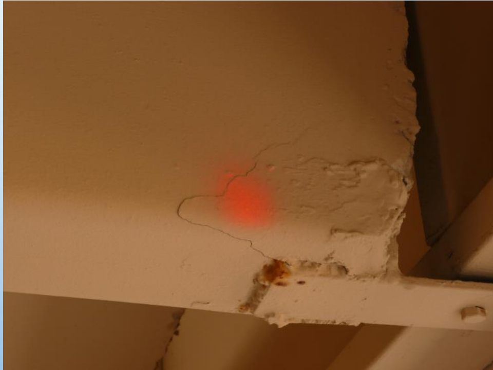
Concrete about to spall
