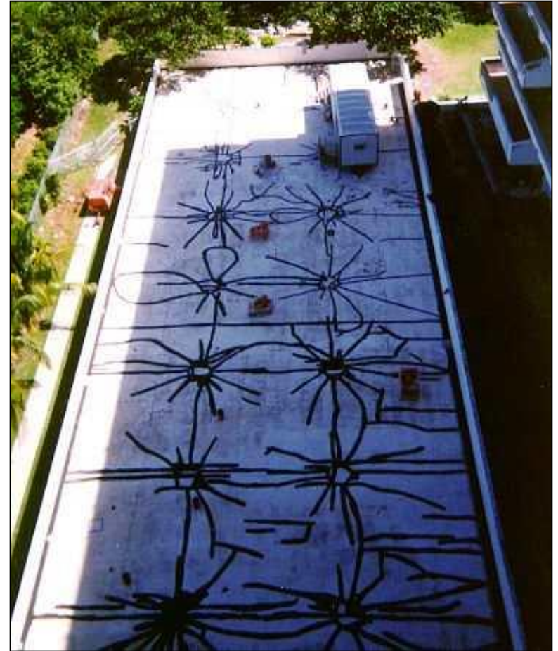
Cracking Pattern on the Roof of a Building with Punching Shear Deficiency (not CH2)
