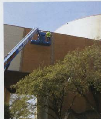
Recoloring of the exterior masonry was carried out using a water-based, penetrating stain composed of a multiple-polymer formulation of resin solids, color pigments, and tint base. Photos courtesy of Nawkaw Corp.
