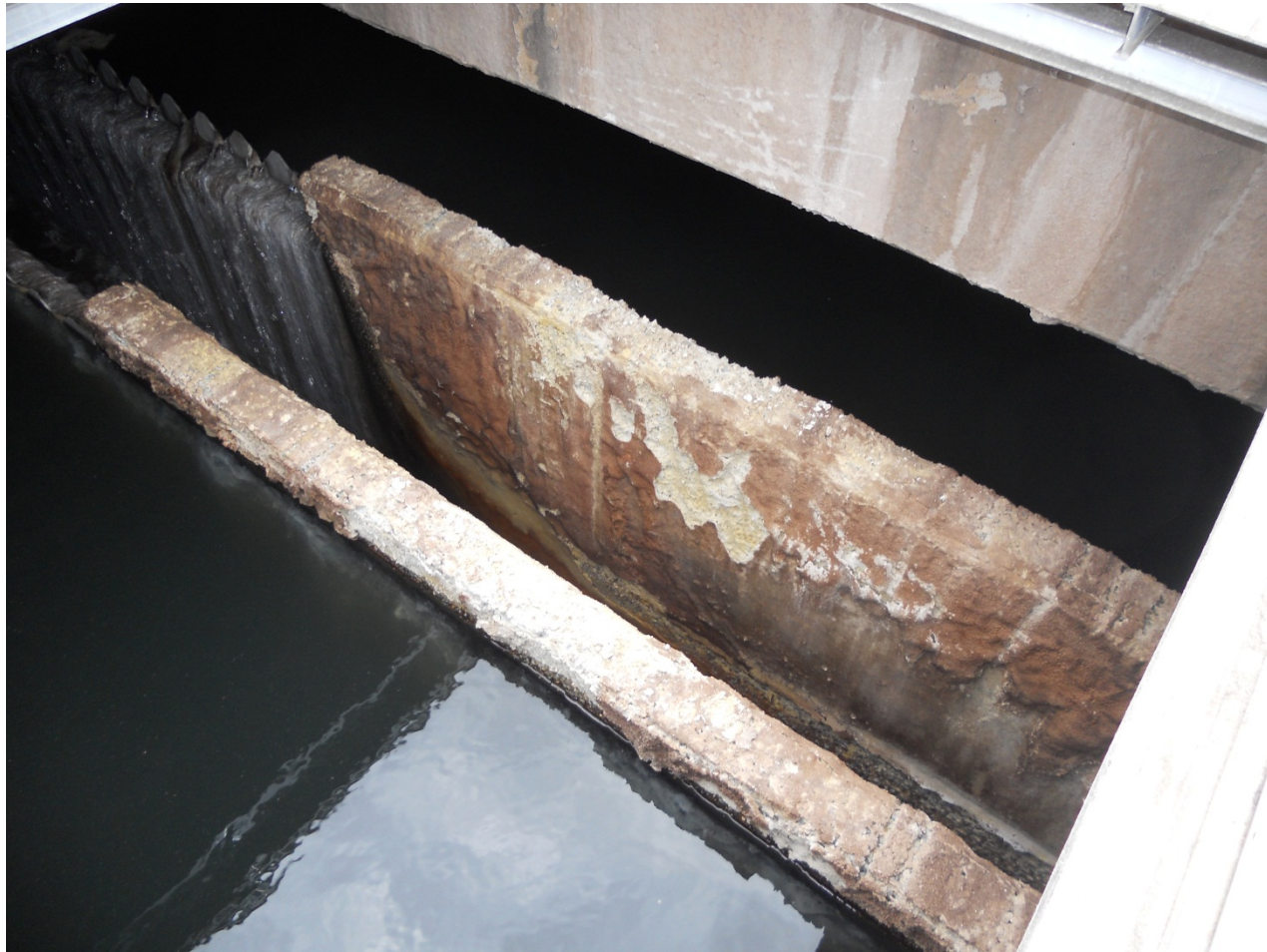
Concrete Corrosion on Exposed Effluent Trough Surfaces
