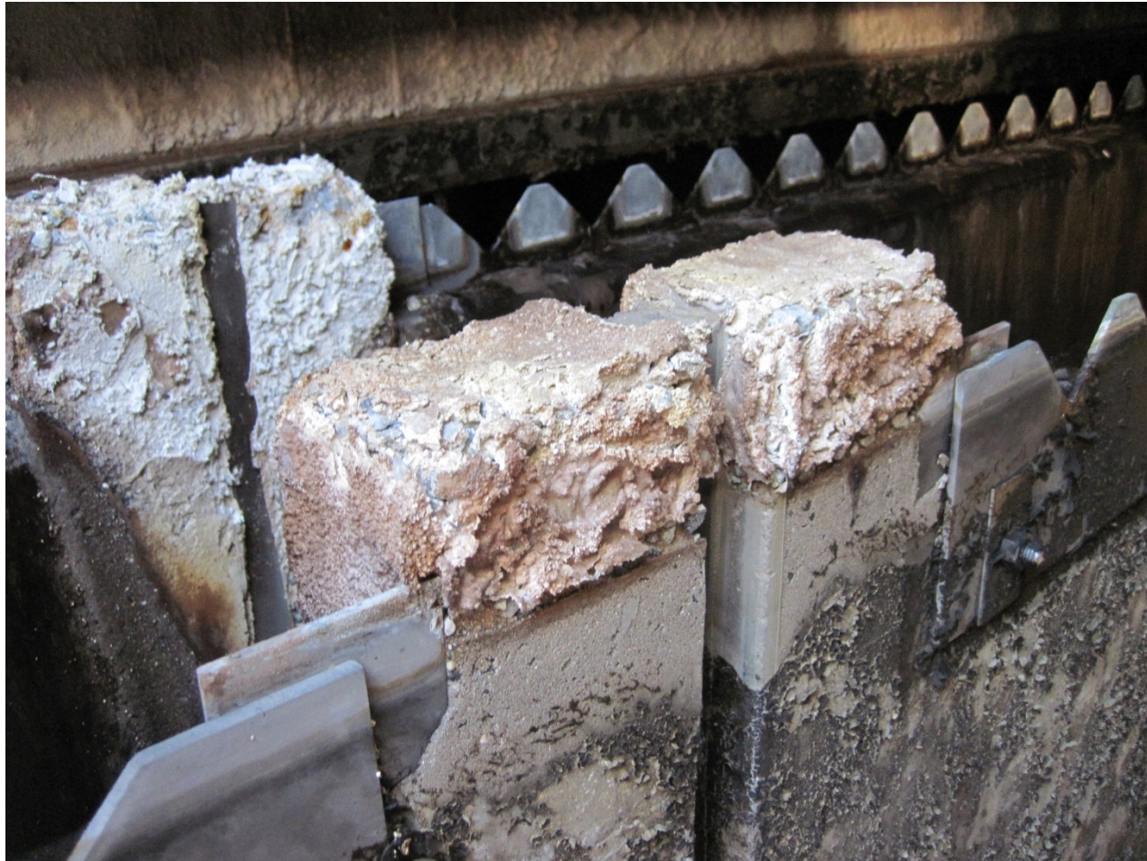
Concrete Corrosion Above Water Level at Adjoining Effluent Trough Segments
