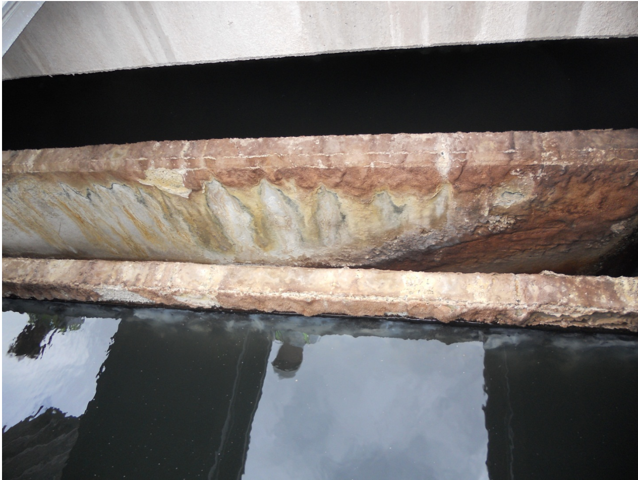
Concrete Corrosion on Exposed Effluent Trough Surfaces
