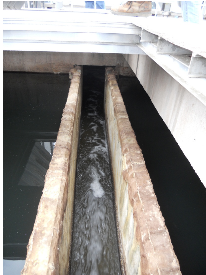
Concrete Corrosion at Effluent End of Trough
