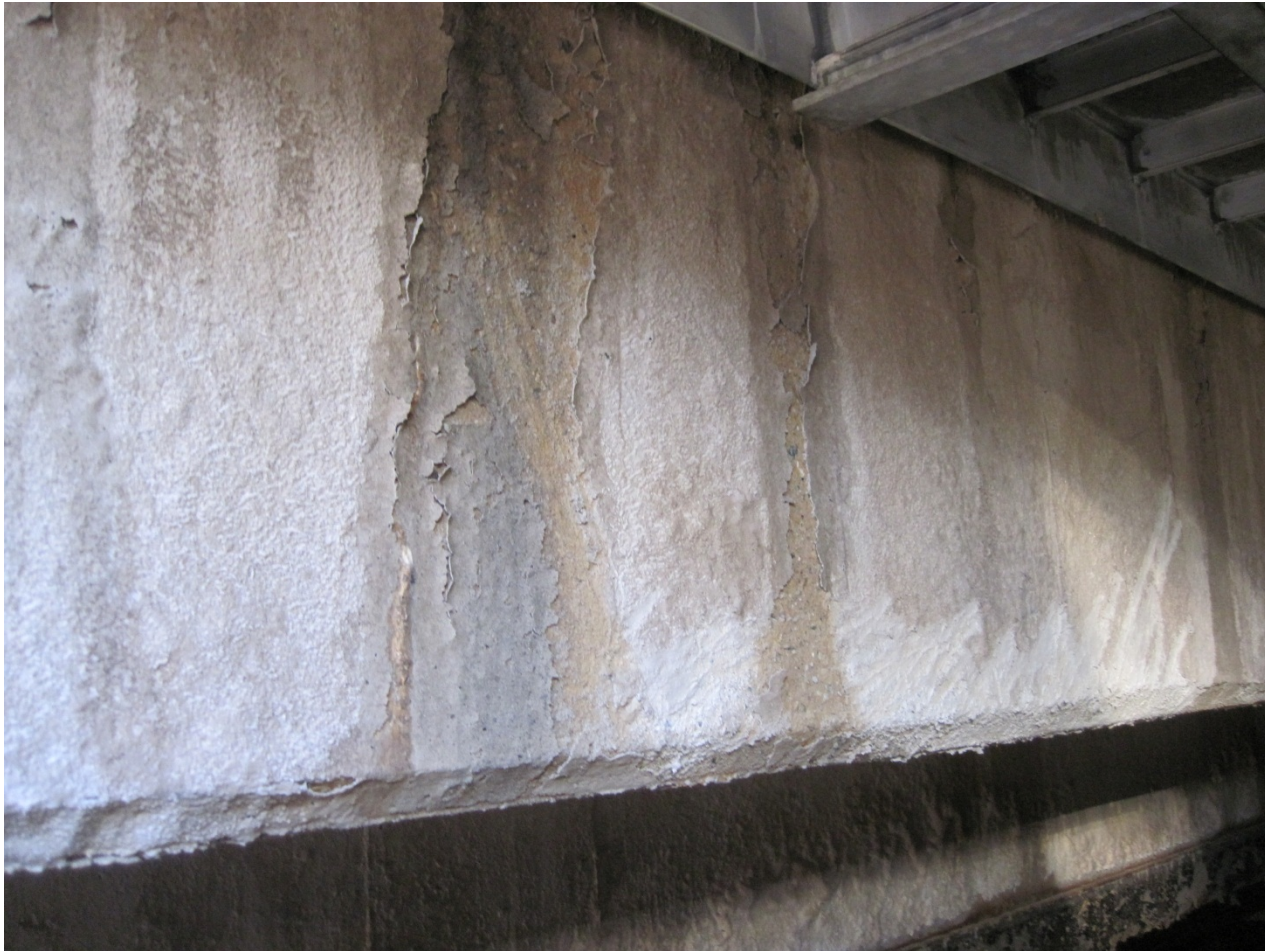
Corrosion of Concrete Over Covered Tank
