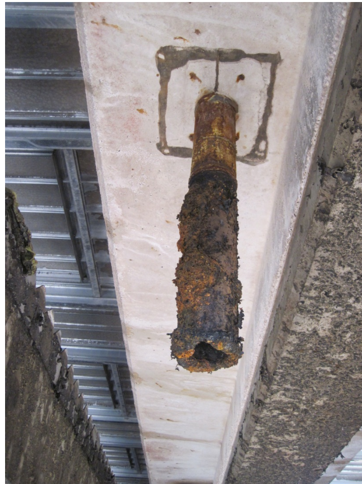
Corroded Drain Pipe
