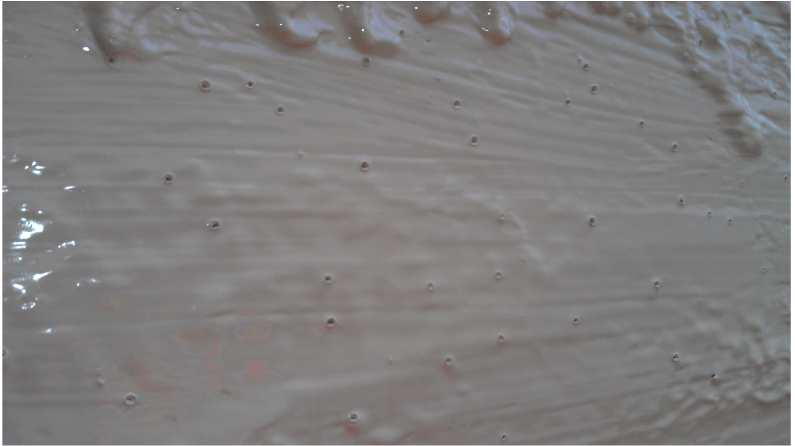
Pinholes in sealer coating.
