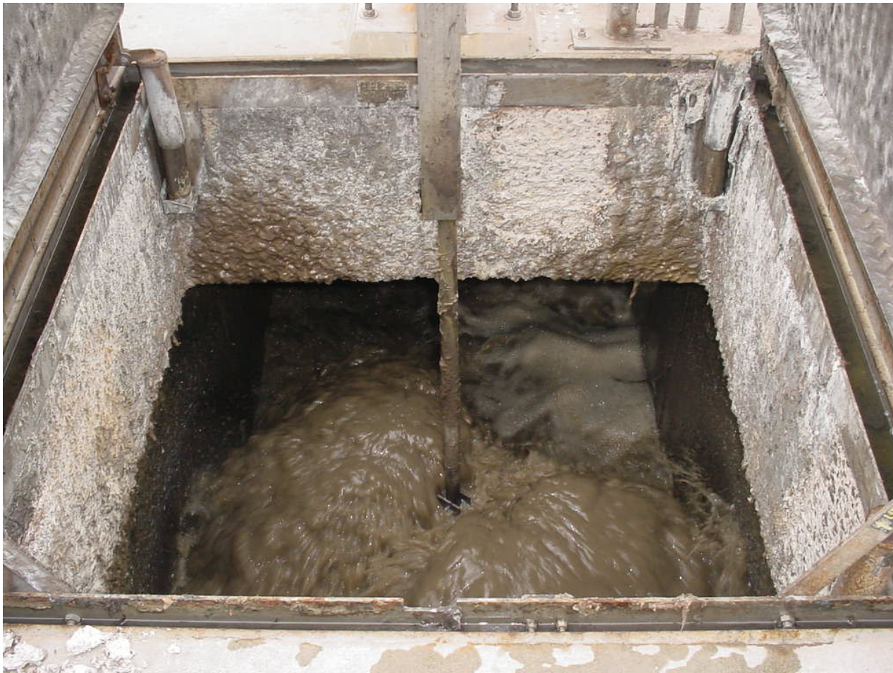
Concrete Corrosion in Sludge Valve Box
