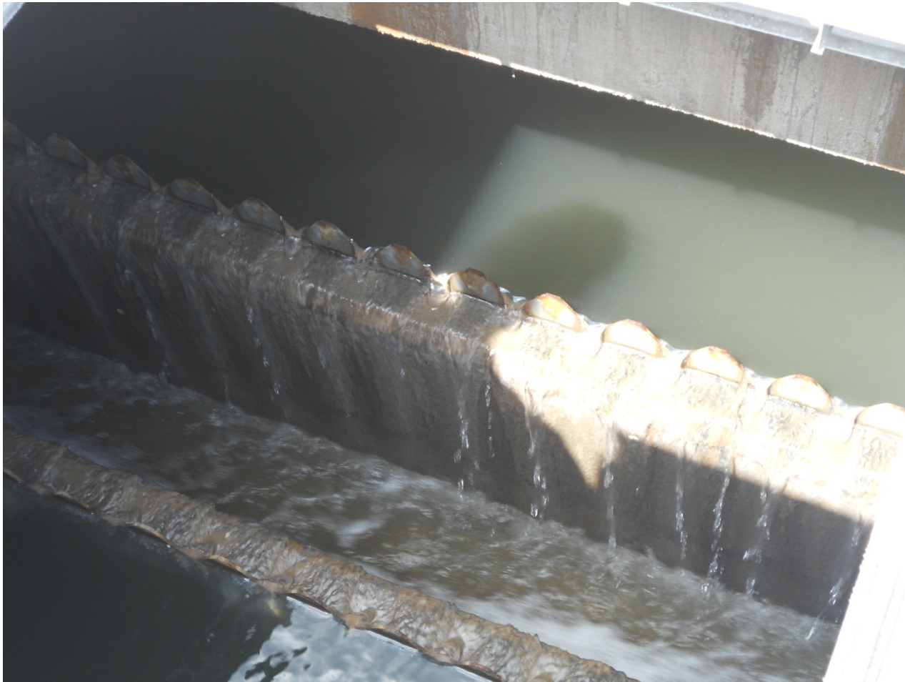
Water Flowing Over Weirs into Effluent Trough
