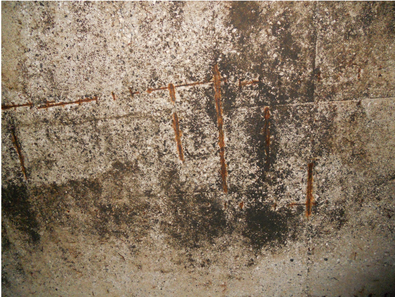
Spalled concrete With Exposed Rebars on Underside of Effluent Channel
