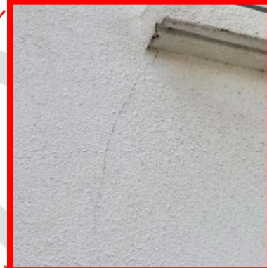
Photo 2.3.17-2: Crack at Bottom of Window
