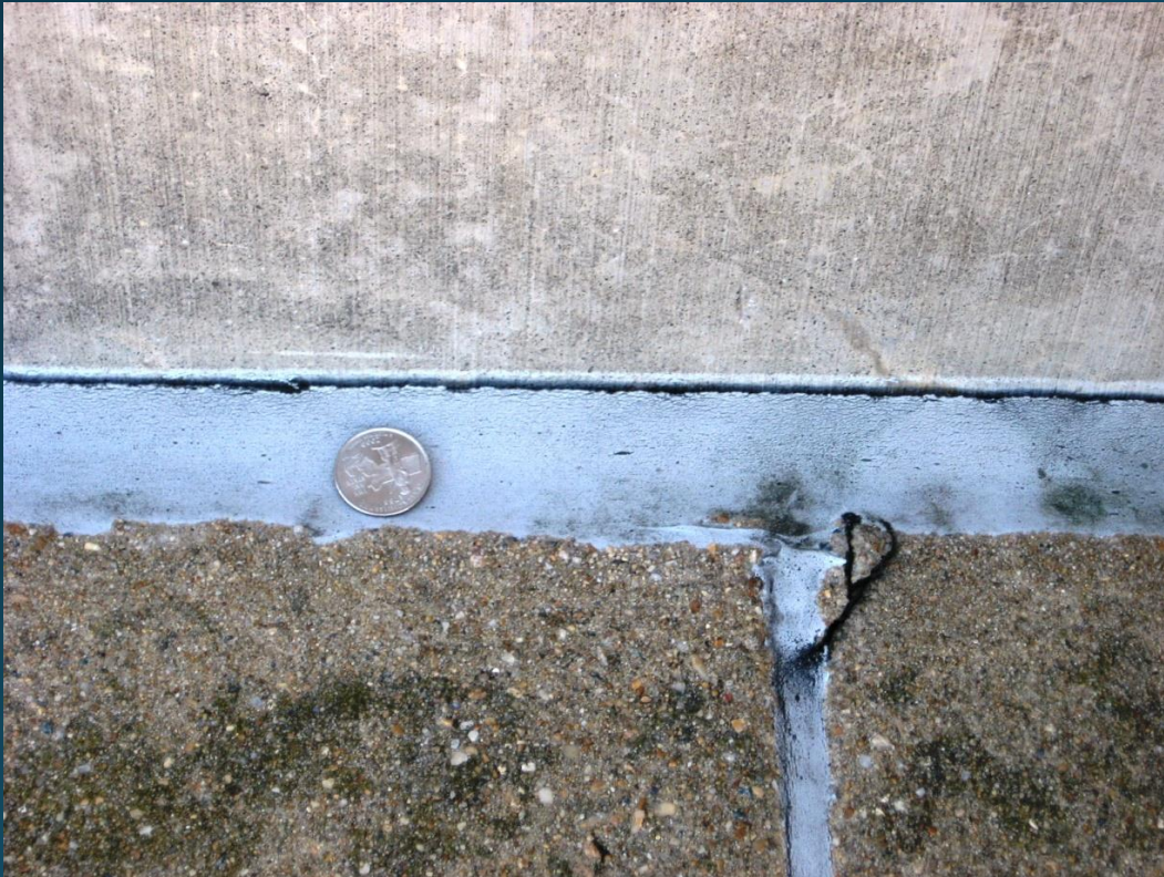
Breach at wall to slab transition joint
