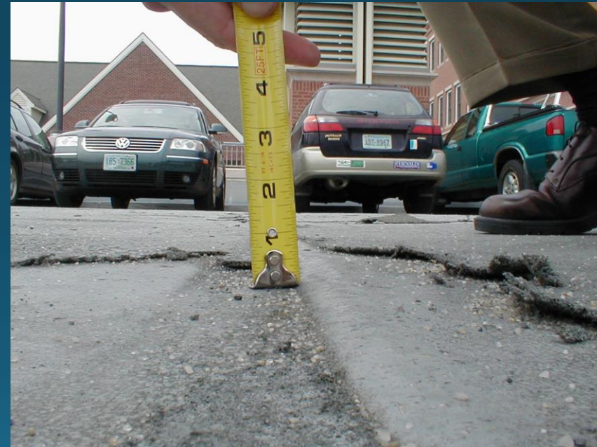
Damage at impact point
