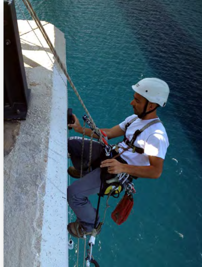
Substrate humidity measurements
