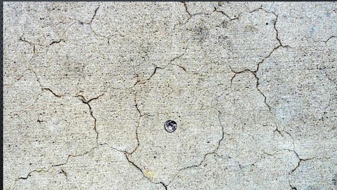
SHRINKAGE CRACKS OR CRAZING
