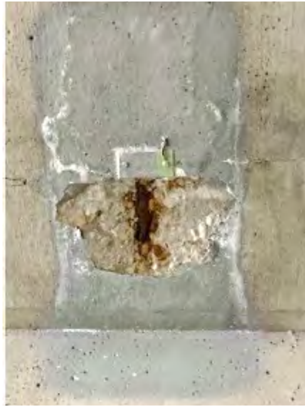
Spalled Concrete in the Metalized Area Showing Corroding Rebar
