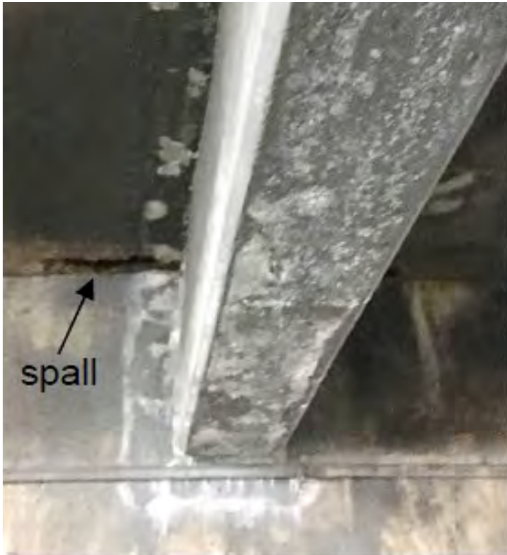
Spalling around CP System White Zinc Oxide Film from corrosion of ZAS
