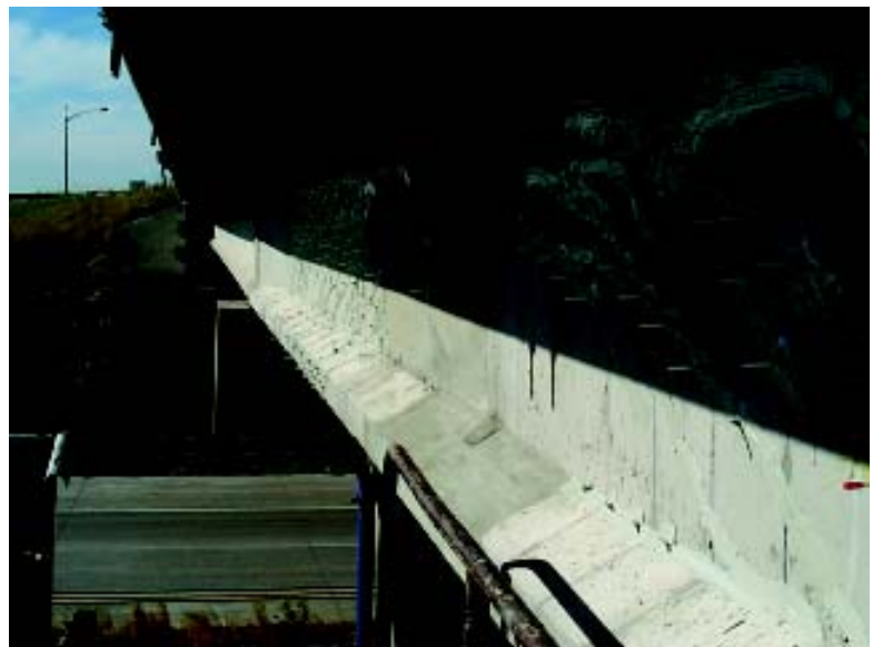
Fig. 3: The damaged girder with injection ports in place
