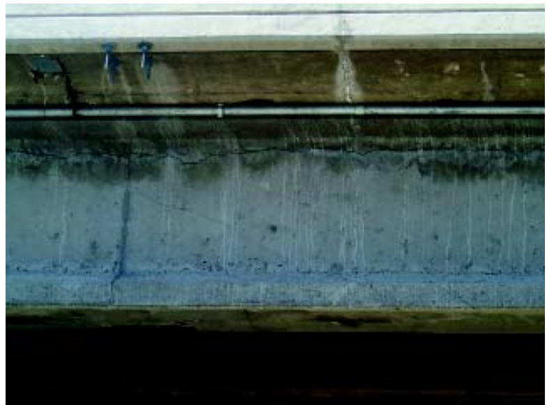
Fig. 2: The damaged girder prior to epoxy injection repairs
