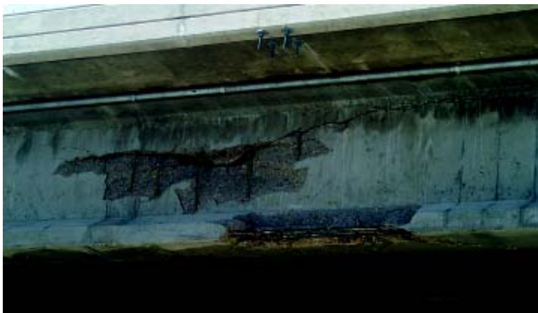
Fig. 1: Damage on the eastmost concrete girder before the repairs
