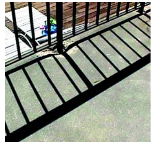
Rail embed spall
