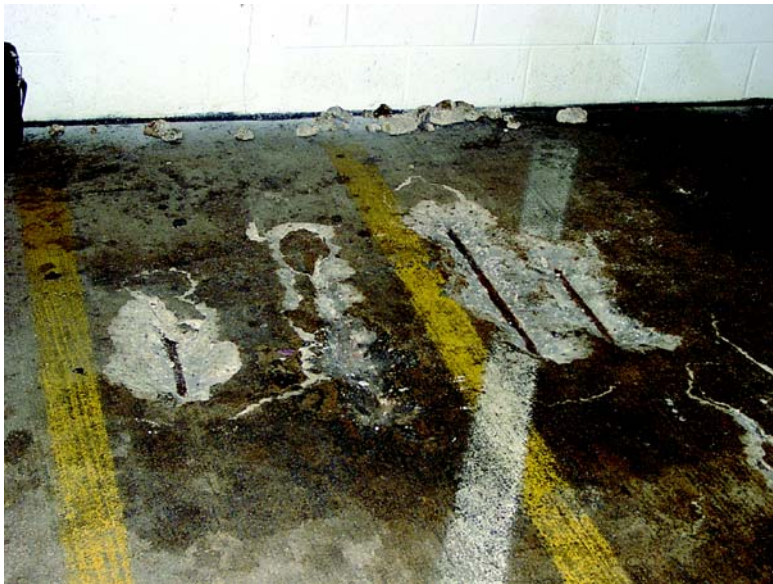
My garage is spalling and breaking up! Is this dangerous?
