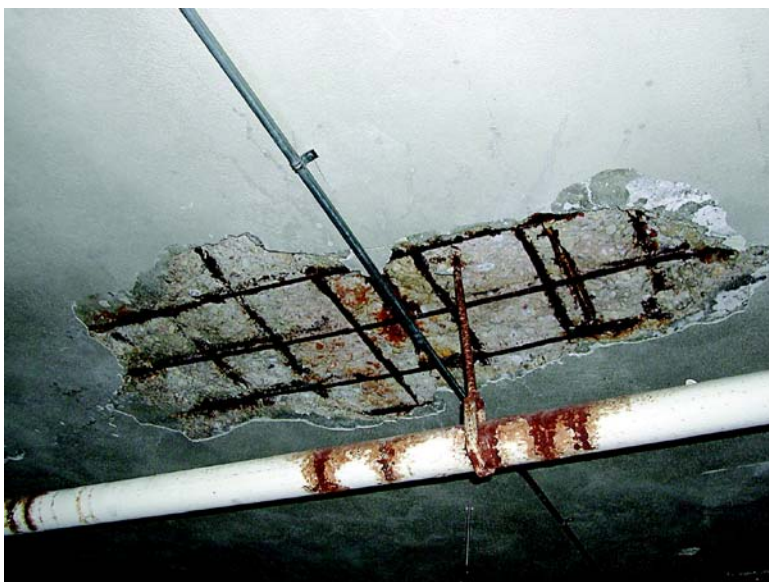
Chunks of concrete are falling from the ceiling. How do I stop this before someone gets hurt?
