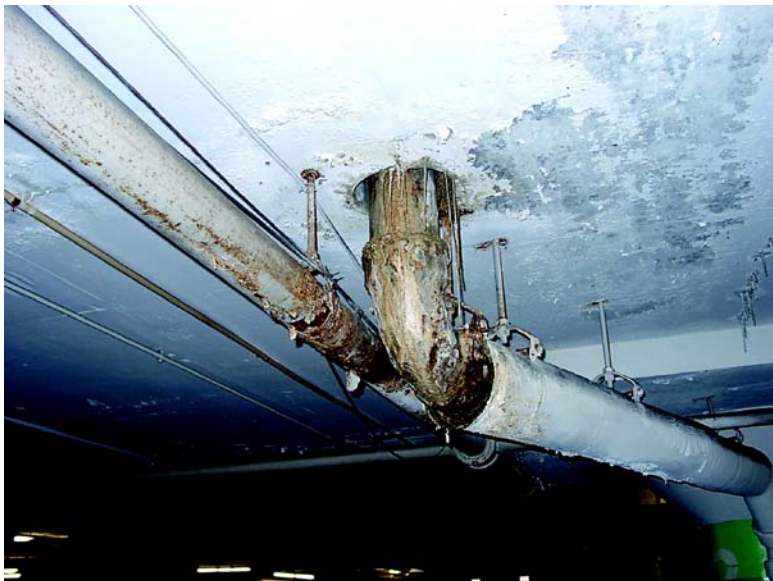
That white stuff is dripping from the concrete and ruining the paint on the cars. What do I do?
