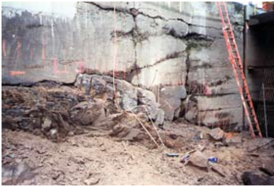
SE forebay wall pre-existing condition, leaning in 8 in. 10 ft (9/27/02).
