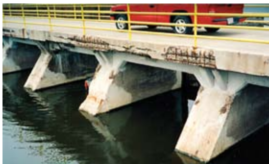
Guardlock bridge deck prior to repairs (4/12/00).
