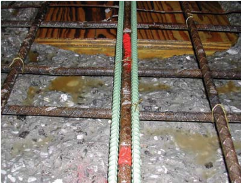
A close-up picture of an existing reinforcing bar spliced with new epoxy-coated bars. Note the section loss on the existing bar due to corrosion.
