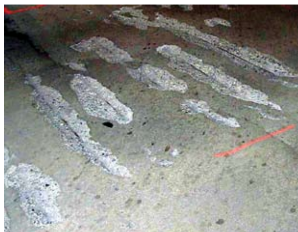
Top surface concrete delaminations and spalls in the waffle slab portion of the garage. The top mat of reinforcing bars can be seen in the spalled areas.
