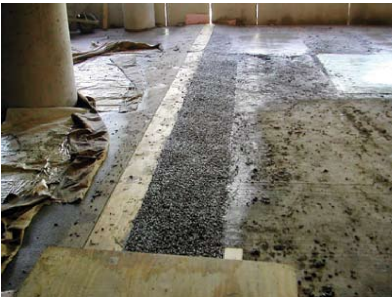
Newly placed concrete in repair areas and along the existing expansion joint. The block out seen in the picture is for the wings of the new expansion joint seal.
