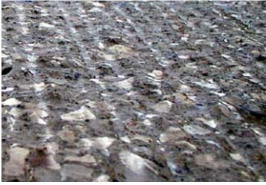
Fig. 3: Surface preparation using a rotomill leaves a smooth surface with aggregate sheared off
