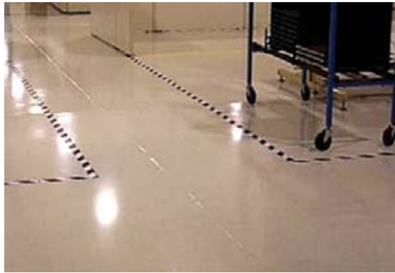
Fig. 2: Extrusion of semi-rigid joint filler due to reverse warping (photo courtesy of Herman Protze)
