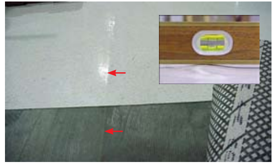
Fig. 8: Debonding and buckling of ESD tile flooring (note hump at arrow and insert)
