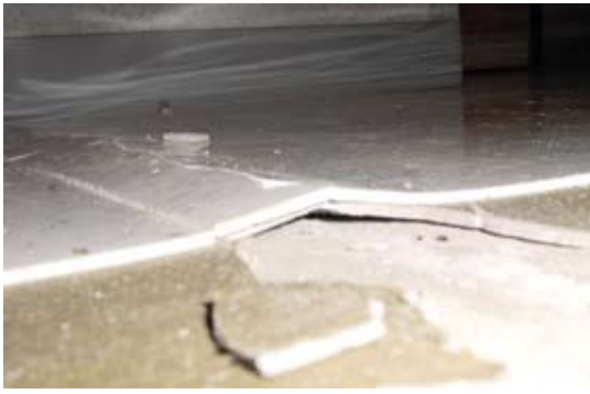
Fig. 1: Buckling of VCT tiles and cementitious underlayment attributed to warping relaxation at concrete slab joints
