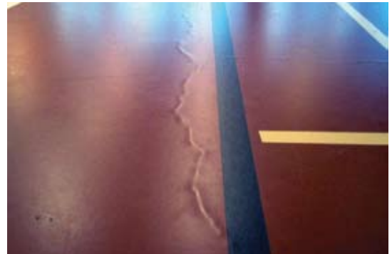
Fig. 9: Extrusion of crack filler beneath poured polyurethane gymnasium flooring
