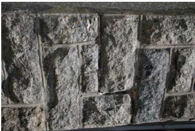
Fig. 1: Typical existing condition at deteriorated masonry joints
