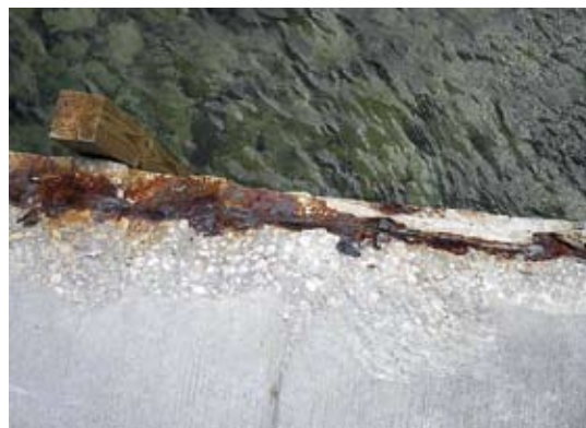
eventually lead to severe damage and extensive repairs
