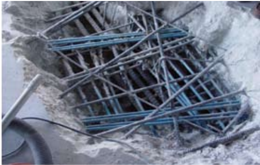
New construction honeycomb/congested reinforcement. Why didn't a standard mixture work here?
