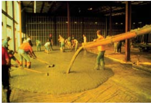
Avoiding poor construction techniques. Where's the mesh?
