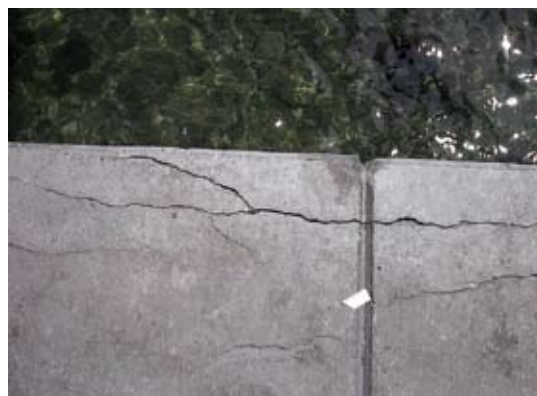
Cracks not addressed...
