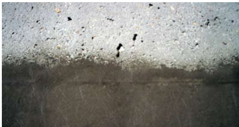
Typical prepared CIP concrete exhibiting bugholes (upper half) and an epoxy modified cementitious overlay applied to create a contiguous surface for lining (lower half)
