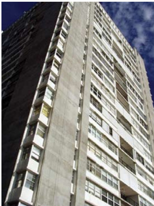
Building with old finish and deterioration
