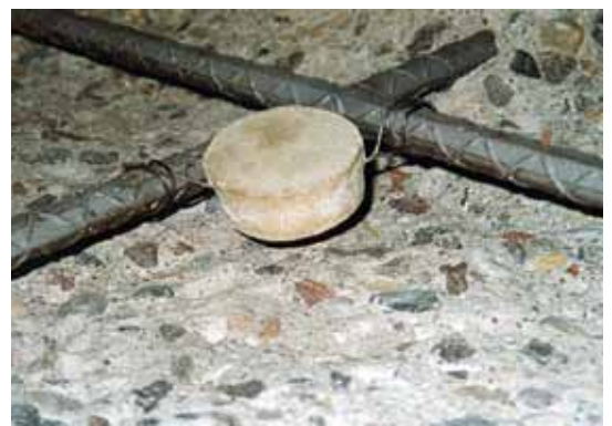
Discrete galvanic anodes are installed along the edge of the concrete patch repair
