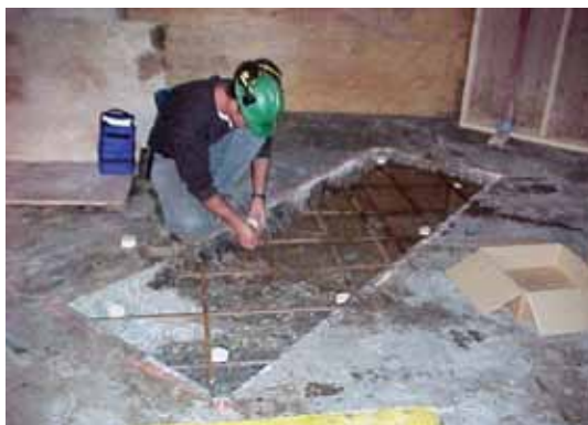
Discrete galvanic anodes installed around concrete repair to provide protection from halo effect corrosion
