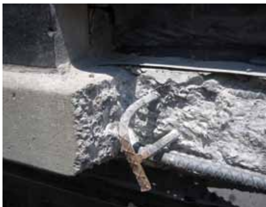
Concrete demolition at exposed slab edge; demolition is nearly complete, surface preparation to follow
