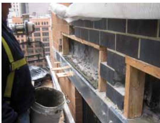
Concrete placement at exposed slab edge. Note the galvanized metal forms fabricated by the repair contractor and shimmed to the brick below to optimize stripping and reforming operations
