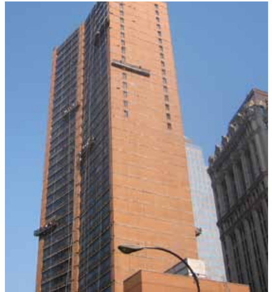
East and south elevations of building under repair in August 2007. Up to 10 swing stages were used during the course of repairs
