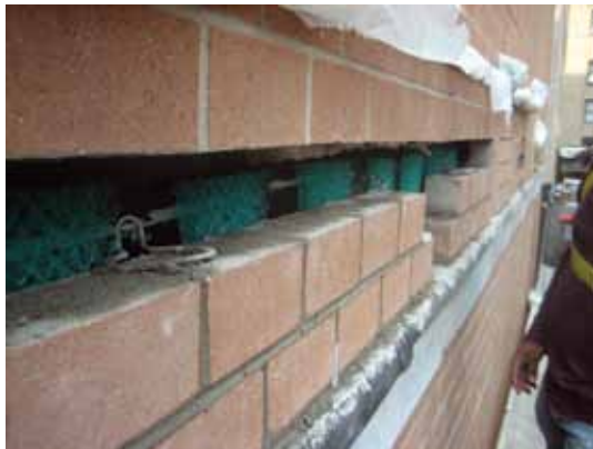
Flashing installation is complete. Brick installation in progress along with cavity netting protecting brick ties and weeps
