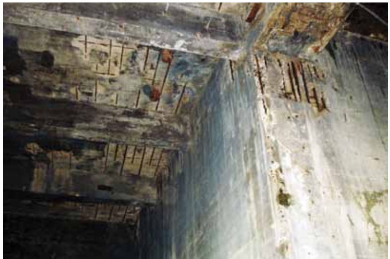
View of interior second floor conditions during selective demolition and repair work. Note moisture damage to wall finishes and soffit (not slab) deterioration
