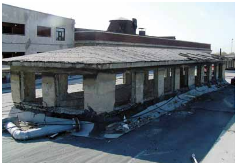
View of one of the two clerestories on the roof that were repaired and restored
