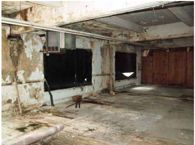
View of basement level soffit and walls that are severely delaminated from embedded reinforcing steel corrosion. Note encased structural steel "I" beams
