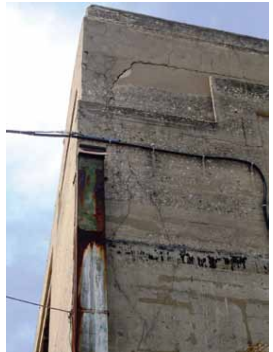
Exterior view of southeast corner of building illustrating concrete façade delaminations and cracks that were repaired
