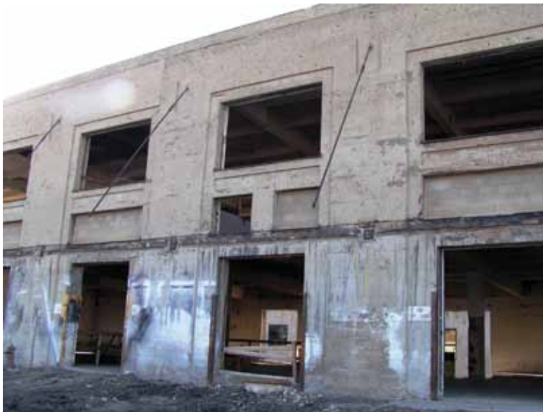
Completed foundation wall delamination repair preparation, ready for form-and-pour repair concrete to complete area
