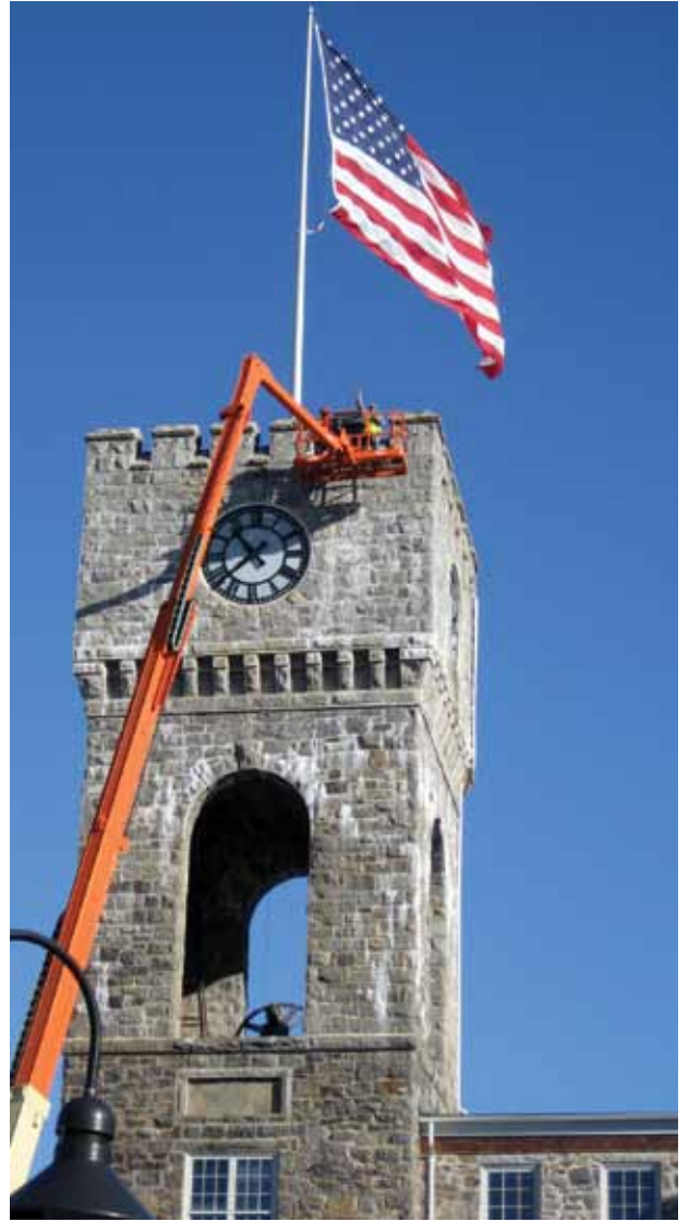
Extensive waterproofing and repair work was needed to revive the old mill
