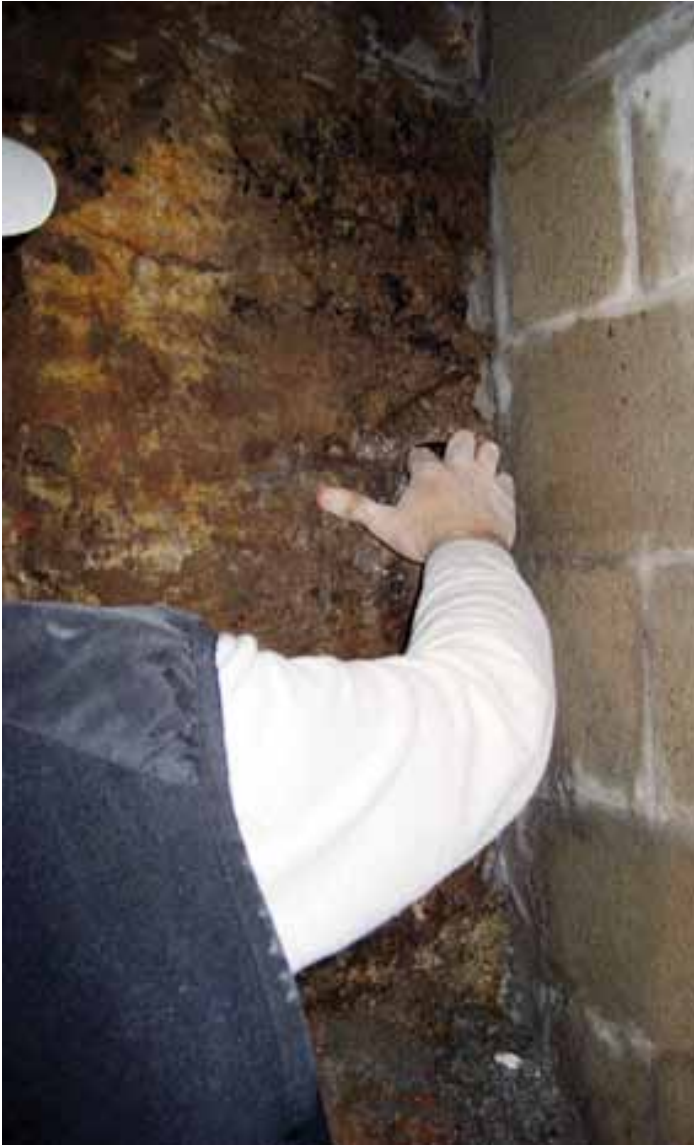
Crack repair was needed in elevator pits
