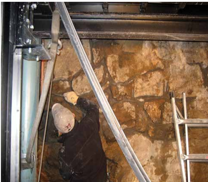
Extensive rubble elevator wall crack repair allowed the facility to pass inspection from authorities
