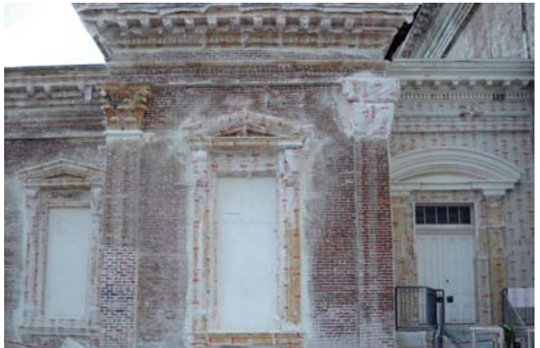
As doors and windows were removed to be repaired, openings were filled to prevent moisture infiltration
