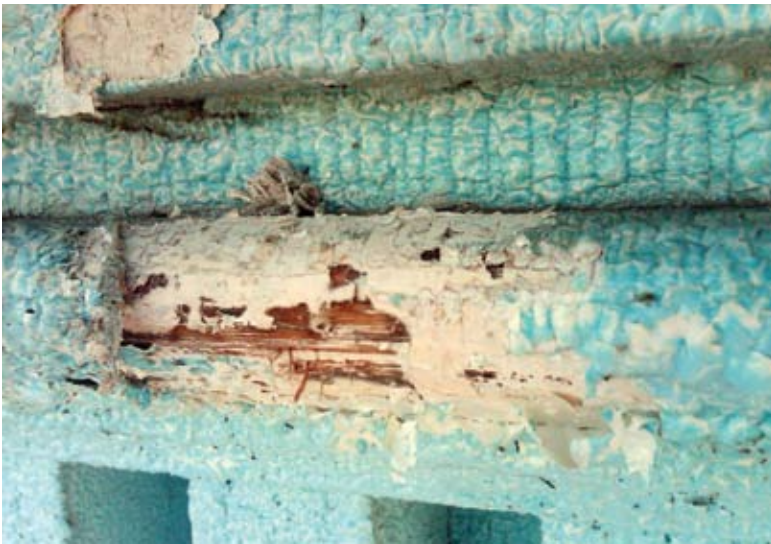
The specified paint removal product was ineffective against the unexpected 0.25 in. (6.4 mm) thick existing lead coatings
