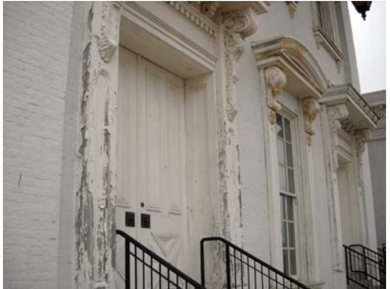
Typical deteriorated coating
