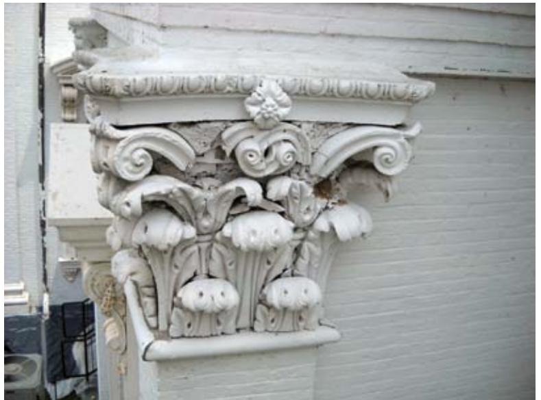
Typical deteriorated capital
