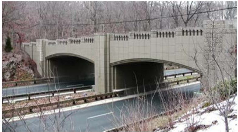
Fig. 1: An historic concrete bridge on the Merritt Parkway in Connecticut coated with an acrylic elastomeric coating custom-matched to the original concrete color. The coating was applied over residual graffiti and previous coatings after their substantial removal
