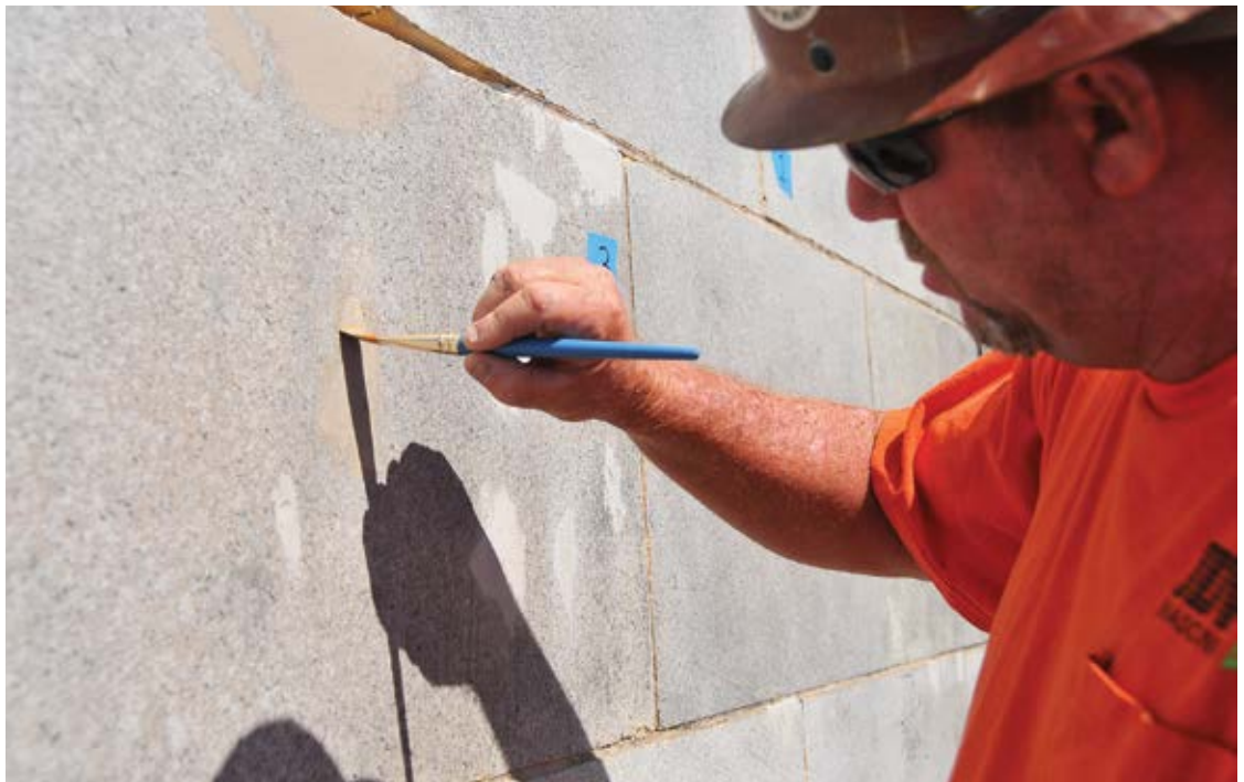
Fig. 2: Worker applies custom-matched aliphatic polyurethane coating to terra-cotta glaze repairs at the California State Library in Sacramento, CA
