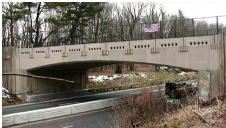
Fig. 3: A replacement span between two remaining historic concrete piers on another Merritt Parkway bridge coated with a color-matched potassium silicate mineral coating
