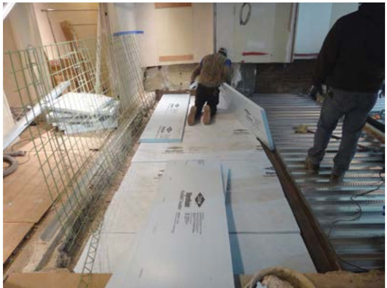
Fig. 9: Unbonded topping slab repair area (with foam filler) adjacent to full-depth repair area on composite metal deck
