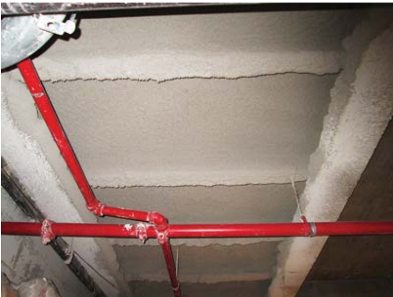
Fig. 11: Closely spaced channels of supplemental support repair (shown after spray-on fireproofing was applied)
