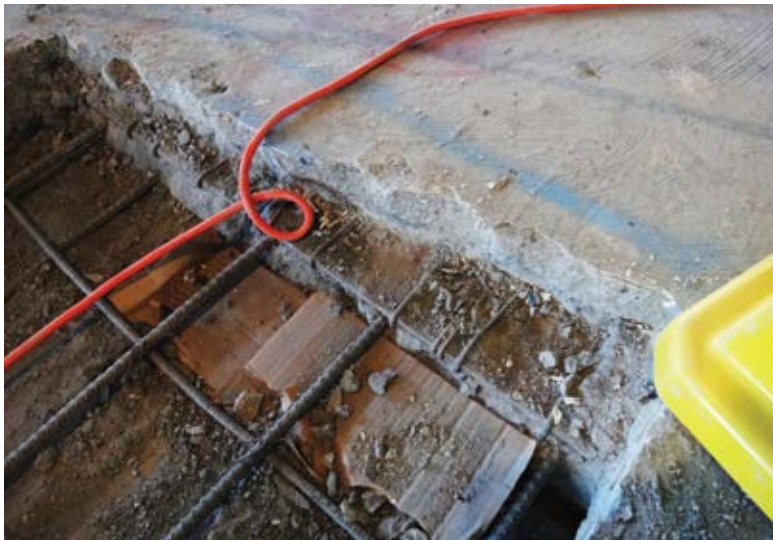
Fig. 1: Typical method of mesh anchorage where welded wire reinforcement is bent and hooked around beam flange
