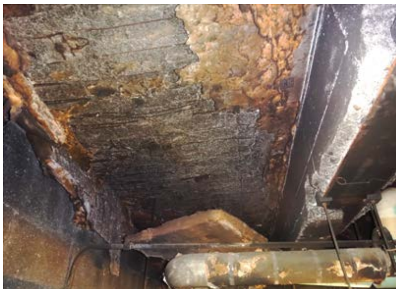
Fig. 3: Deterioration of slab due to corroded reinforcement at slab underside
