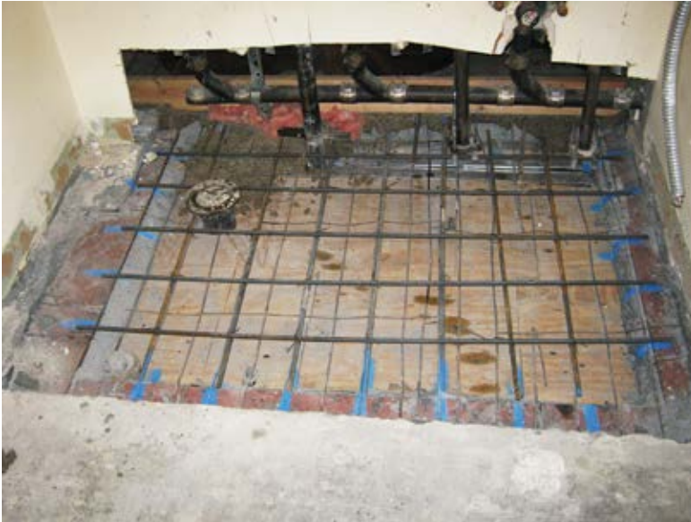
Fig. 10: Full-depth repair area with existing reinforcement and new additional reinforcement placed on wood formwork
