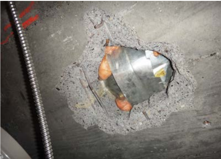
Fig. 6: Existing poorly executed repair made at a full-depth penetration
