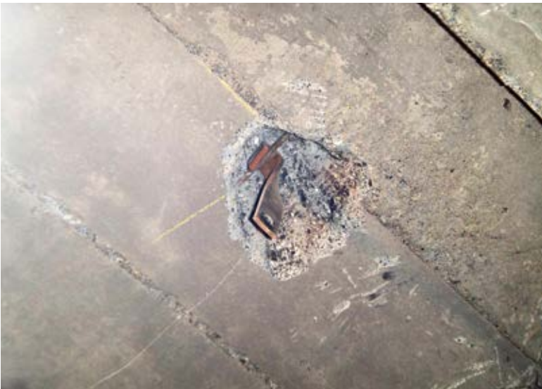
Fig. 7: Partial-depth slab damage where a wire of the reinforcement was exposed and used for supporting a hanger
