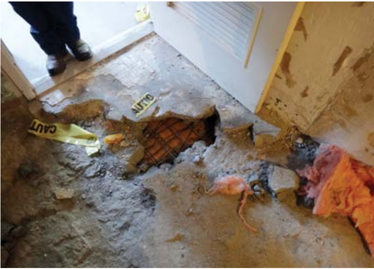
Fig. 5: Partial-depth and full-depth slab damage from finish removal during a tenant fit-out
