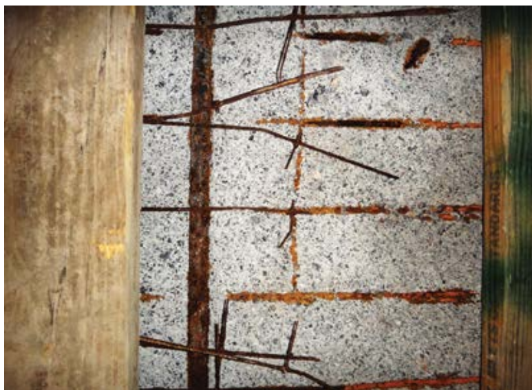
Fig. 4: Close-up view of corroded reinforcement at slab underside
