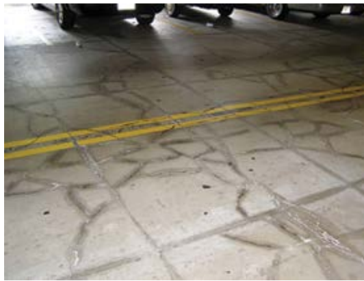
Fig. 2: Cracking and concrete spalling of topping slab (plaza deck system)
