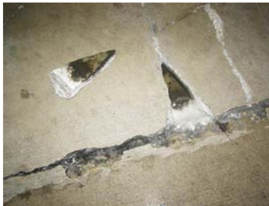
Fig. 3: Lack of bond at waterproofing membrane caused delamination and spalling of concrete segments in topping slab between cracks
