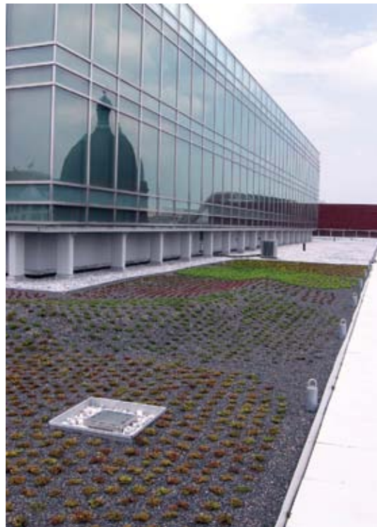
Completed green roof at 1225 Connecticut Avenue in downtown Washington, DC. The project helped the owner attain LEED Platinum rating
