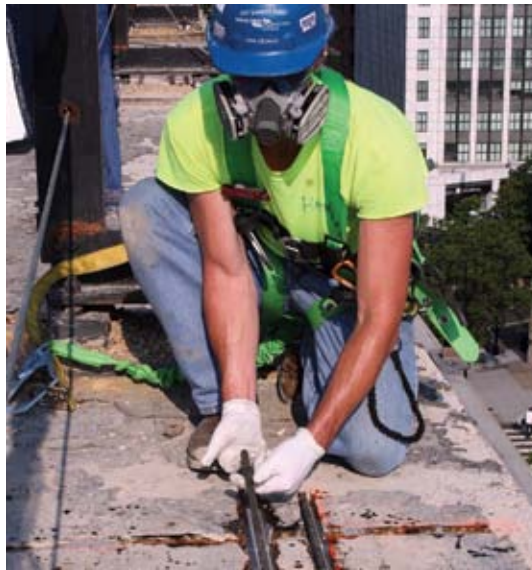
Installation of NSM carbon rods on the top side of the slab
