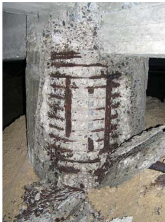
Fig. 7: Column with severe damage (red condition)
