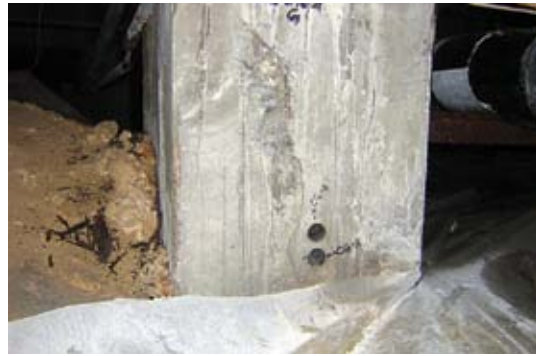
Fig. 5: Column with minor damage (yellow condition)
