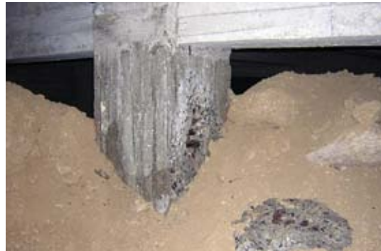
Fig. 6: Column with intermediate damage (blue condition)
