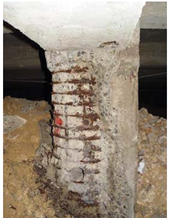
Fig. 3: Corrosion damage to the crawl-space columns
