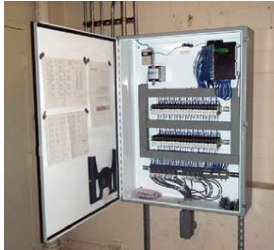
Fig. 10: Monitoring cabinet in central location
