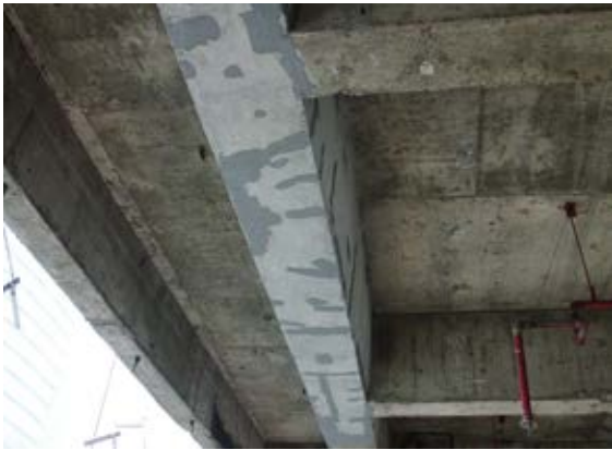
Fig. 10: Patched air voids on beam
