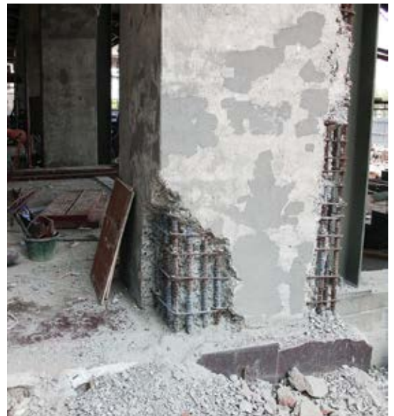
Fig. 8: Poorly consolidated concrete found on column
