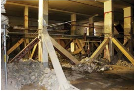
Fig. 2: Steel bracing members installed prior to concrete removal at core walls, columns, and perimeter walls. Plywood sheathing was applied to protect steel members from damage during the construction demolition process
