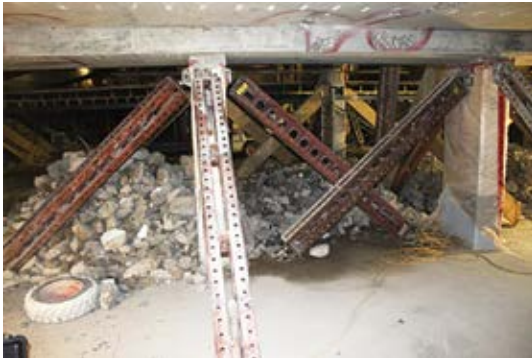
Fig. 3: Typical column bracing along demolition phasing boundary. Demolition debris was stockpiled on slab-on-ground during some phases of work
