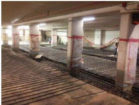
Fig. 9: Forming and placement of new reinforced parking deck floor slab prior to concrete placement
