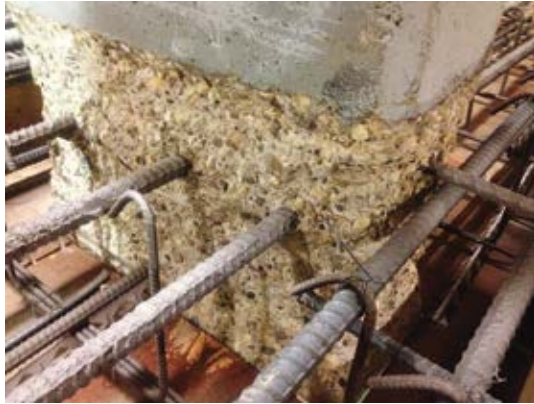
Fig. 8: Existing slab and slab-band reinforcing steel were maintained, abrasive-blast cleaned, and reincorporated into the new work at the perimeter walls, core walls, and interior columns
