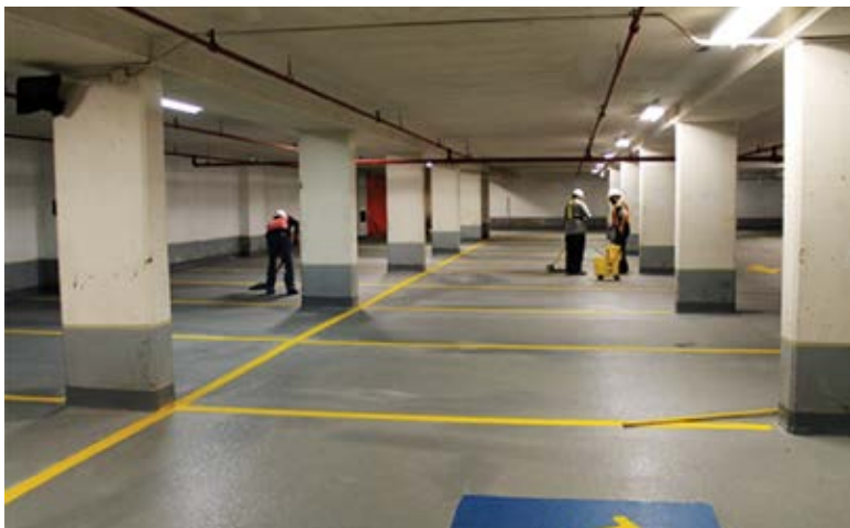
Fig. 10: Highly durable protective coating and sealant materials were used on the new parking deck floor slab surface
