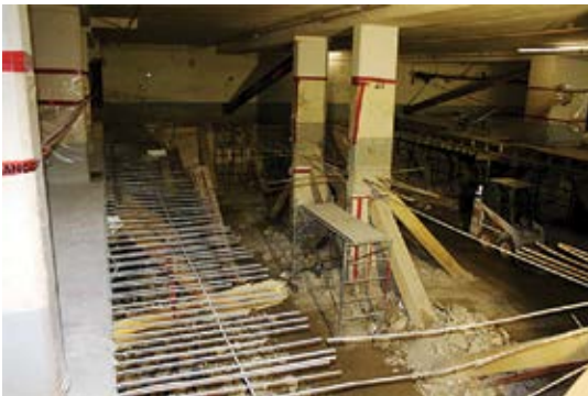
Fig. 7: Slab removal and replacement operations were carefully sequenced over several phases to maintain lateral support for the building walls and columns, while minimizing bracing and shoring requirements
