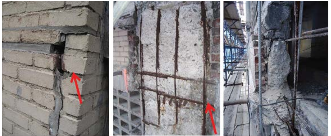
Fig. 7: Concrete deterioration at some columns required full-depth replacement. Red arrows identify approximately the same location
