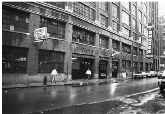
Fig. 4: Shoppers Garage (undated, ca. 1975) showing façade deterioration (Photo courtesy of the City of Boston Landmarks/ Archaeology Photostream on www.flickr.com)
