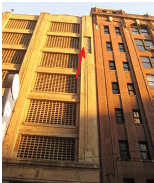
Fig. 6: A panel of brick veneer fell from the façade on October 8, 2011
