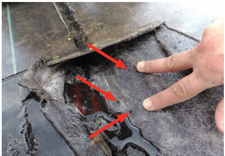
Fig. 8: Breaches in waterproofing membrane detected with LVELD through undamaged protection board
