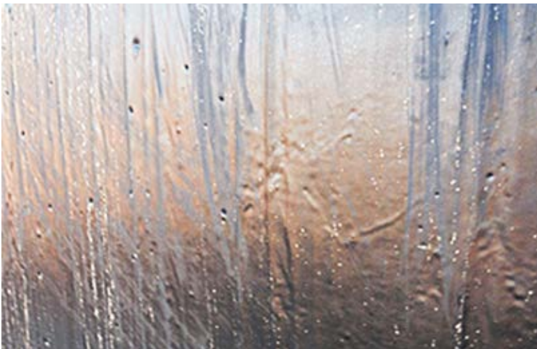
Fig. 4: Pinholes observed on vertical surface
