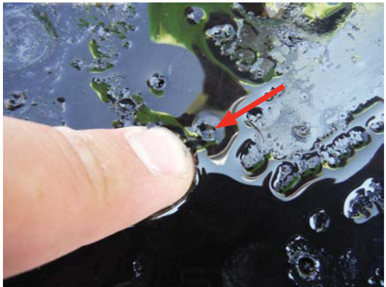
Fig. 7: Pinhole detected with LVELD
