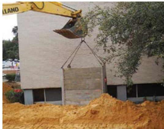
Fig. 6: Trench boxes were placed in the narrow excavation at The Black Academy of Arts Building to allow for safe completion of the repairs in the limited areas where shoring or benching was not a possibility
