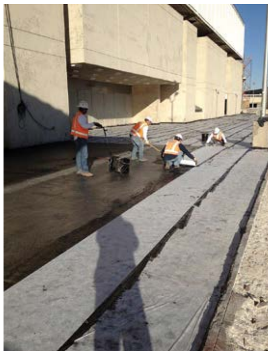
Fig. 2: A geotextile reinforcing fabric was applied between layers of the hot fluid rubberized waterproofing
