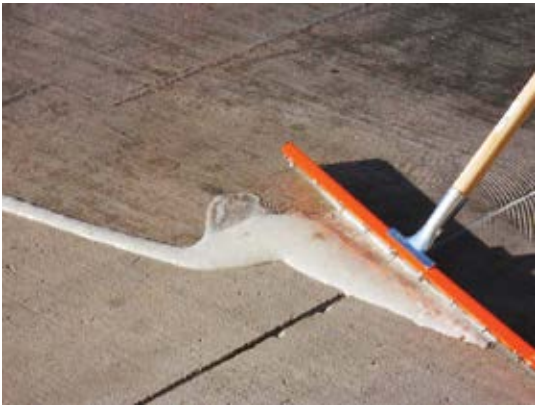
Fig. 3: A low-modulus epoxy resin binder was applied to the loading dock to allow for movement of the substrate and withstand the heavy traffic sustained during multiple events at the convention center
