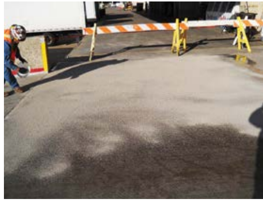
Fig. 4: An aggregate broadcast was applied into the epoxy coating for slip resistance
