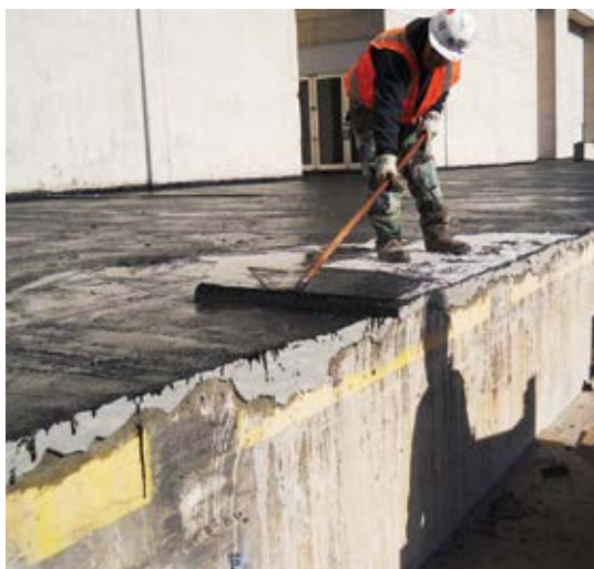
Fig. 1: Hot fluid rubberized waterproofing was applied at approximately 450°F (232°C) to achieve a 90 mil (0.09 in.) layer
