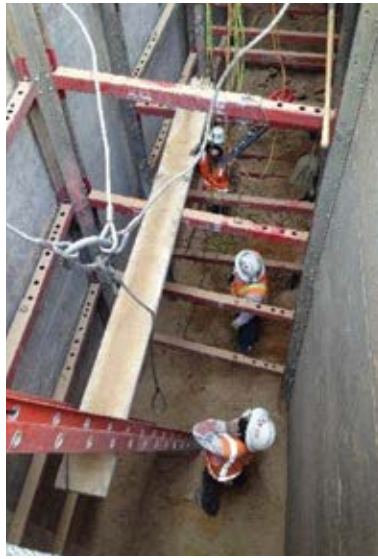
Fig. 8: The crew worked safely in the trench box to apply the below-grade waterproofing to the basement of The Black Academy of Arts Building
