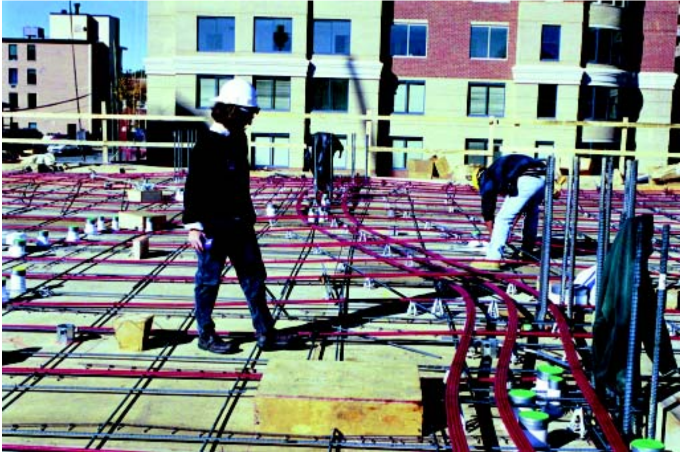
Fig. 1: A 20-story condominium building under construction. Unbonded tendons for a two-way slab are being laid out in a 'banded' configuration. Tendons in one direction are banded over the column lines. Tendons in the other direction are uniformly spaced approximately 3 feet on center
