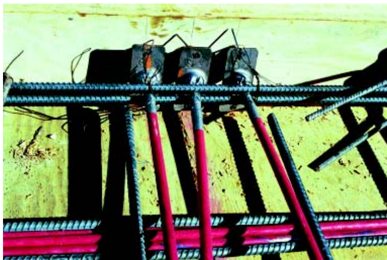
Fig. 2: Stressing-end anchorages of the tendons shown in Fig 1. Since the structure will be enclosed, the tendons are not considered exposed to an aggressive environment; the anchorages are therefore not required to be encapsulated. The ends of the tendons have been taped to avoid exposing the strand
