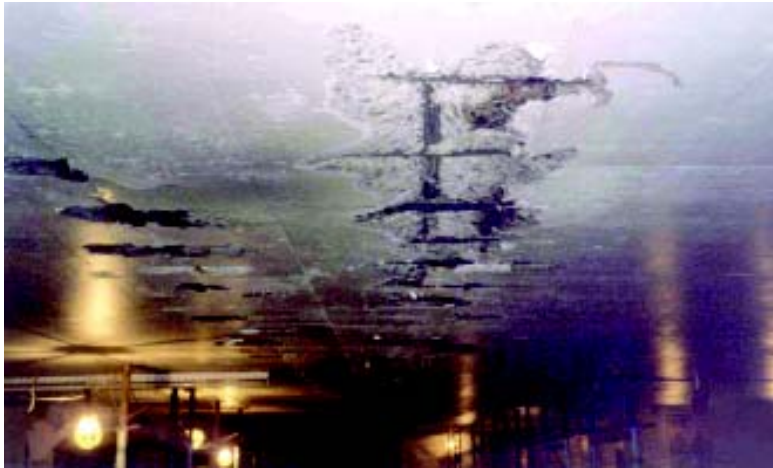
Severely deteriorated concrete soffit
