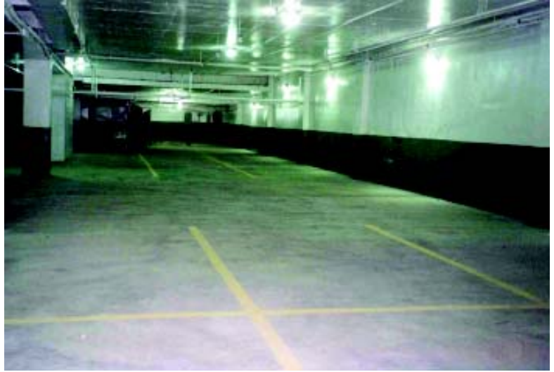
Photo shows replace concrete slab with striping and freshly painted walls and columns
