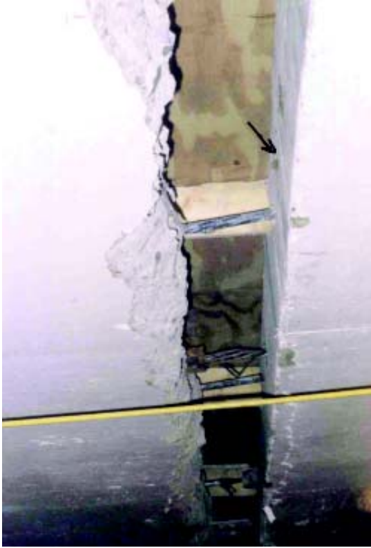
Severely corroded and/or broken PT cables at intermediate stressing location
