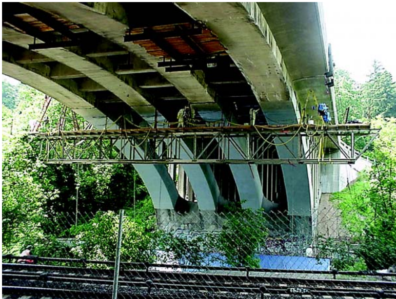
Access to the arches was provided by hanging scaffolding. Application of the composites was performed in 6-ft sections
