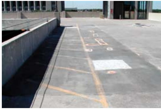
Concrete marked for removal after evaluation
