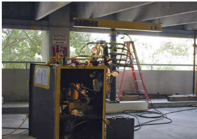
Fig. 3: Jacking equipment used to raise double tee beams during bearing pad replacement
