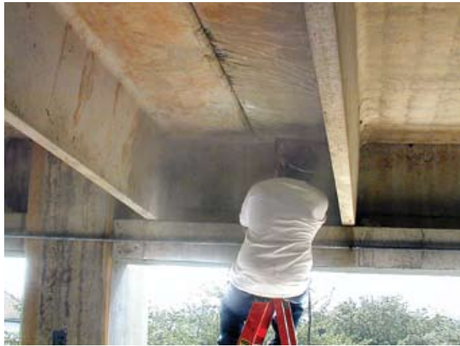
Fig. 1: Expansion joint requiring repair
