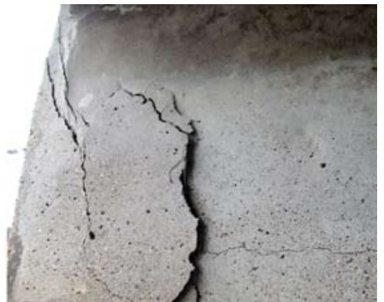
Fig. 2: Concrete repair failure
