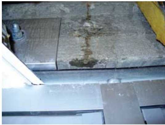
Fig. 7: Same crack leaks
