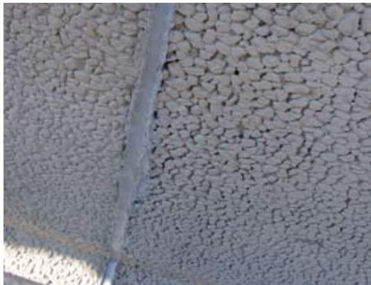
Fig. 2: Vertical joint with gaps in aggregate
