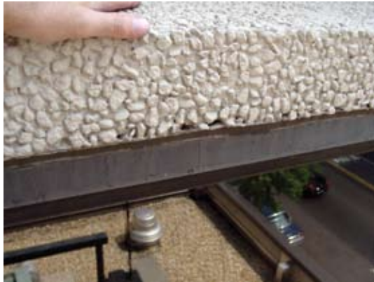
Fig. 1: Horizontal joint with gaps in aggregate
