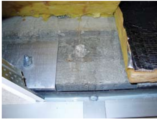
Fig. 6: Vertical crack at connection constraint
