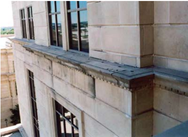
Fig. 2: Heavily soiled cast stone at a water table due to water run-off
