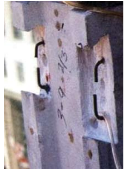
Fig. 12: Preparation for patch repairs. Note the saw cut edges and supplemental anchors to engage the new patch material
