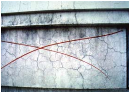
Fig. 3: Heavy crazing in a cast stone façade panel
