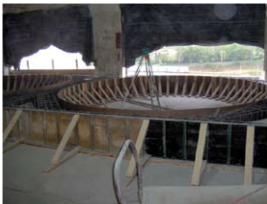
Large diameter tank supports
