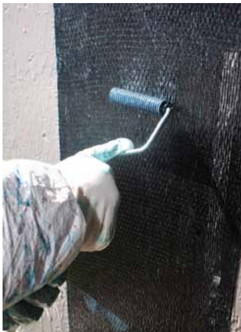
Carbon sheet material is pressed with a ribbed roller to ensure no air bubbles are trapped beneath the fabric
