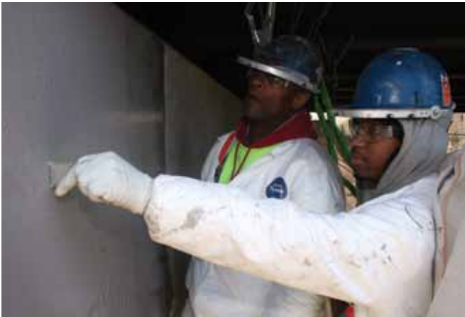
Application and quality control of tack coat prior to placement of carbon sheets
