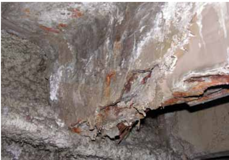
Fig. 1: Double-tee stem deterioration
