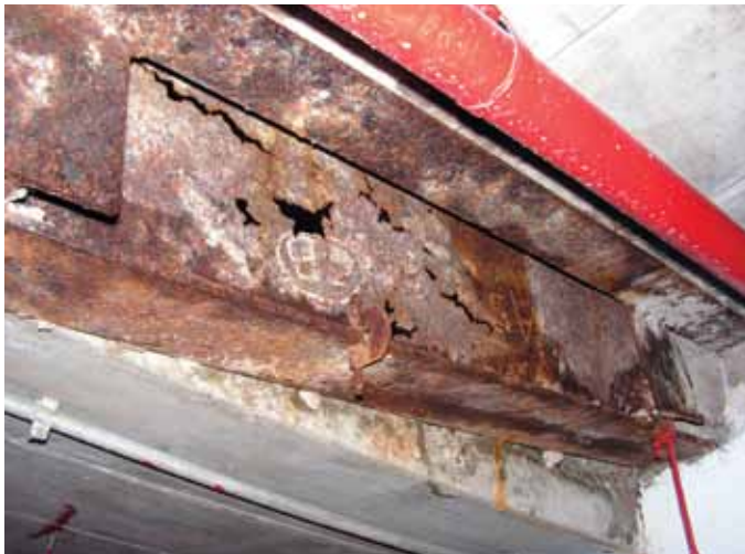
Fig. 5: Steel beam deterioration at ramp
