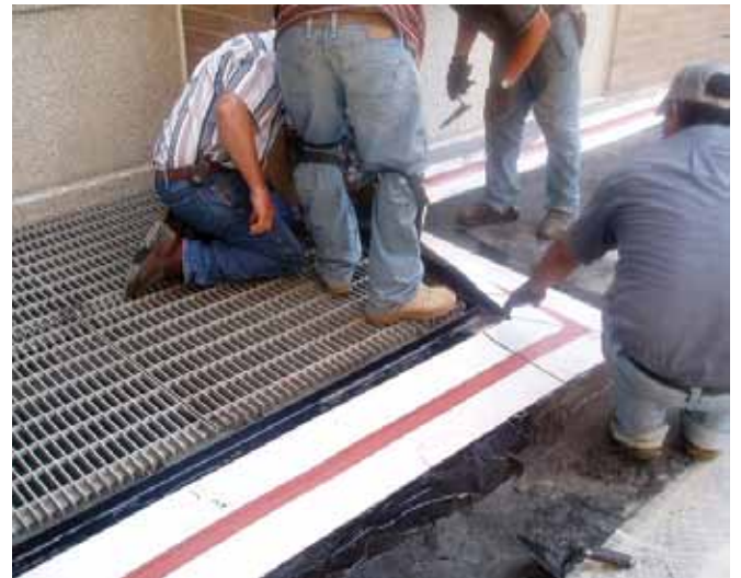
A new waterproof expansion joint system was installed between the plaza level and the building
