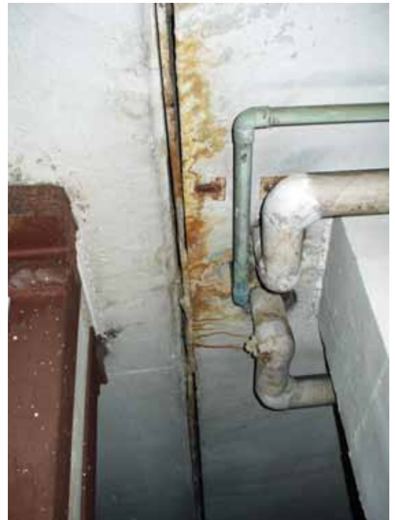
Deterioration and staining due to failure of existing expansion joint
