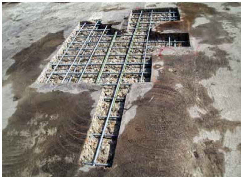
Exposed reinforcement during the predemolition survey and concrete preparation
