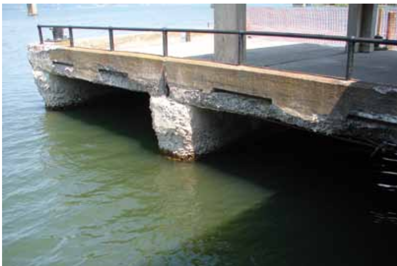
Severe deterioration of concrete due to location on Lake Champlain and harsh climates
