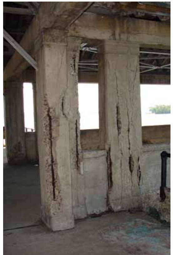
Severe spalling and cracking of concrete columns with exposed reinforcing bar
