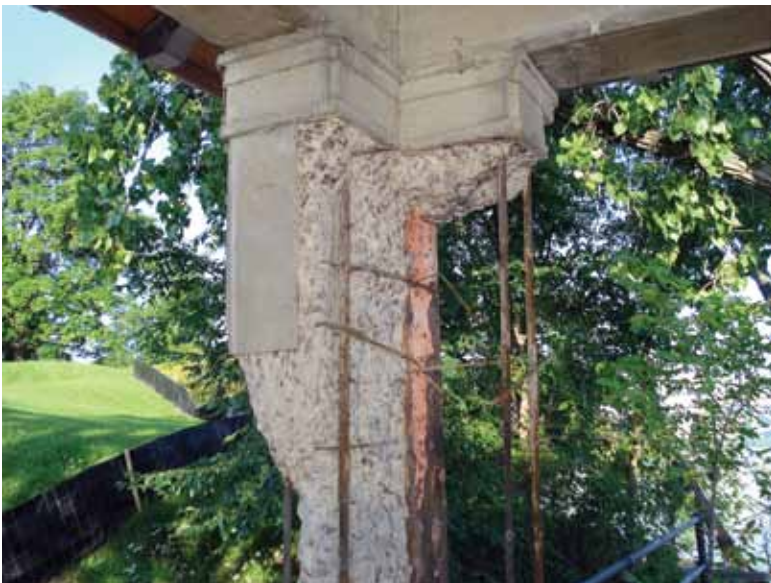
Concrete column after surface preparation. Note the large loss of concrete sections
