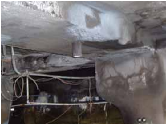
Damage from harsh environment
