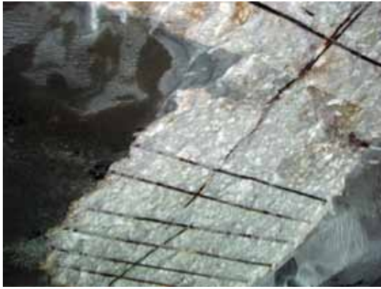
Corrosion on underside of deck
