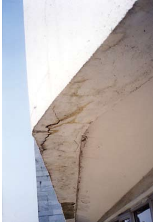
Delamination of façade render with corrosion-induced cracks
