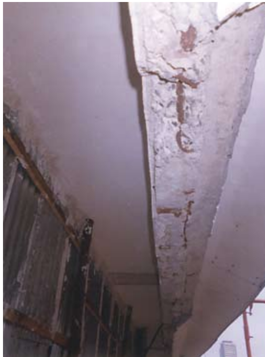
Deterioration in façade concrete elements
